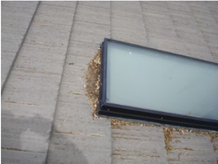
Debris should be removed annually
