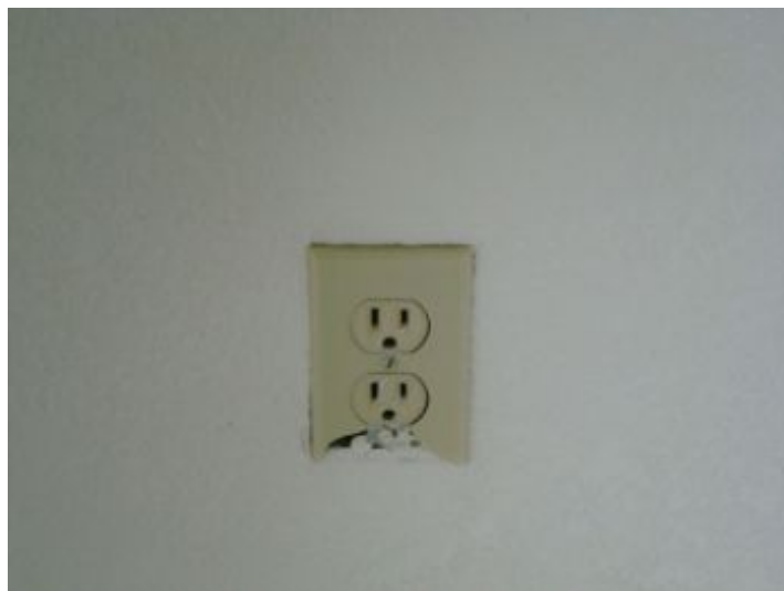
Cover should be replaced.
