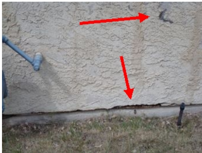
Water damage from sprinklers.
