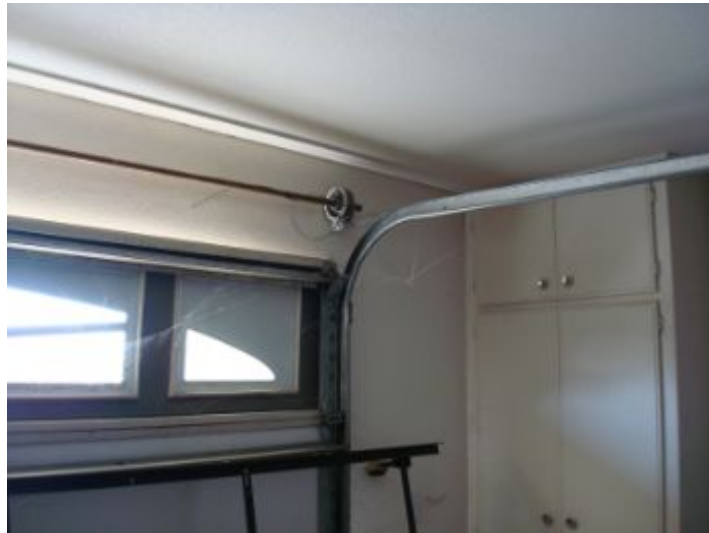
Maintenance repairs needed
