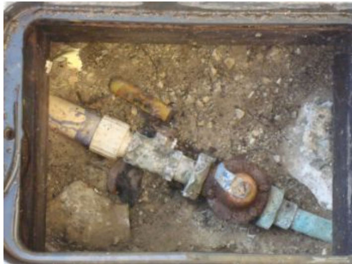
Valve handle broken
