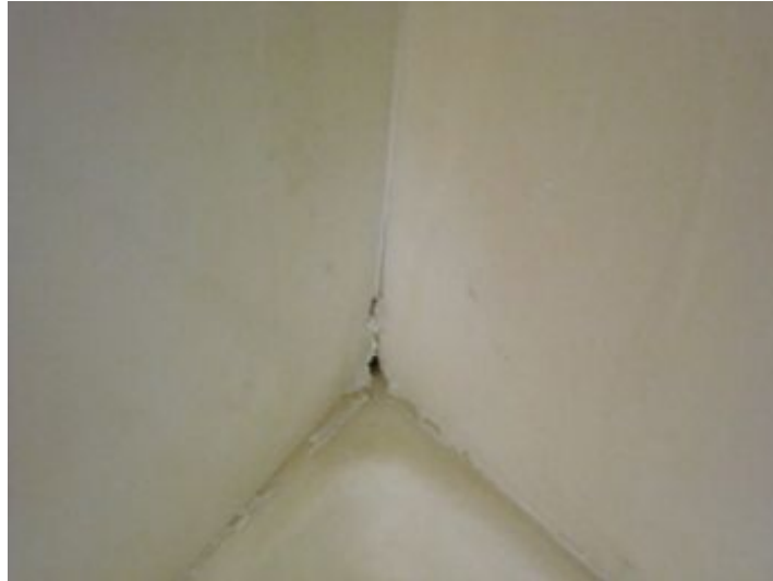
Caulking needed around perimeter.
