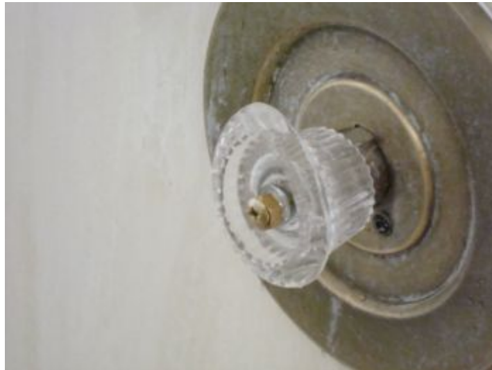
Faucet needs to be replaced
