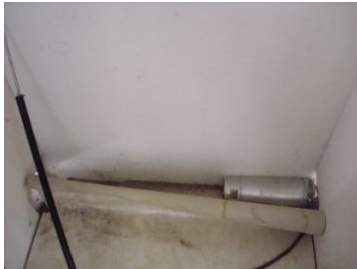
The dryer vent terminates in the garage.
