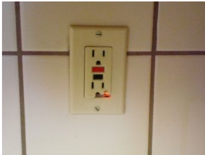
Outlet is broken needs to be replaced
