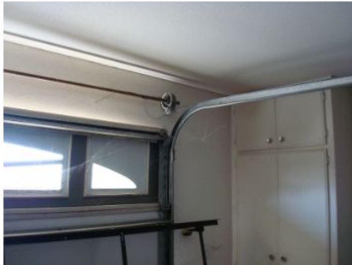
Maintenance repairs needed
