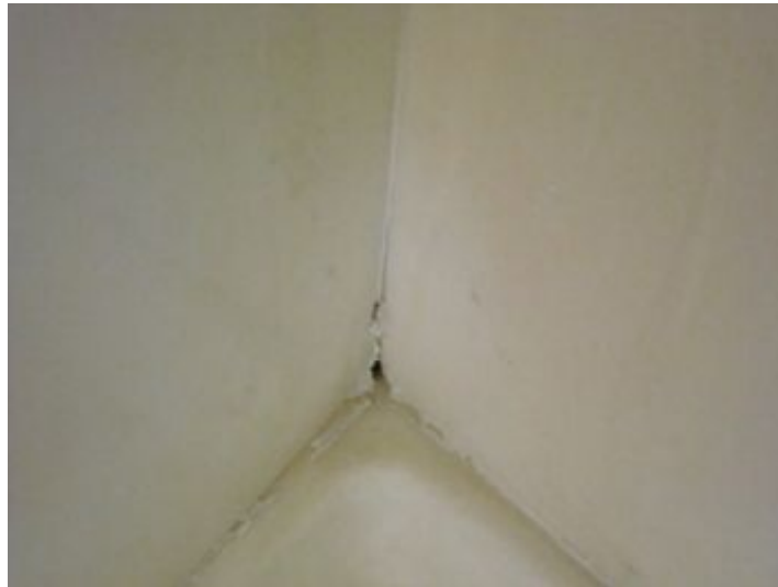
Caulking needed around perimeter.
